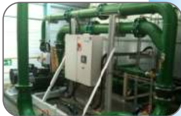
Air Conditioning Plant
